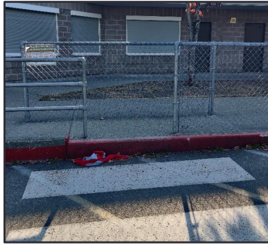
FIGURE 6. CURB LETDOWNS TO CROSSWALK MISSING
